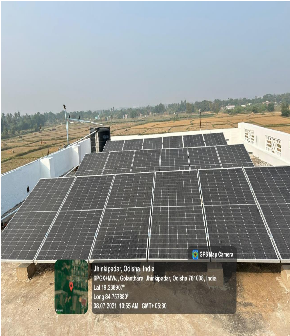
Alternate sources of energy (Solar PV cell)
